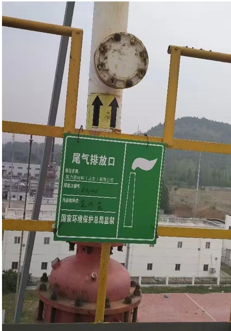
废气检测点标志牌↑
